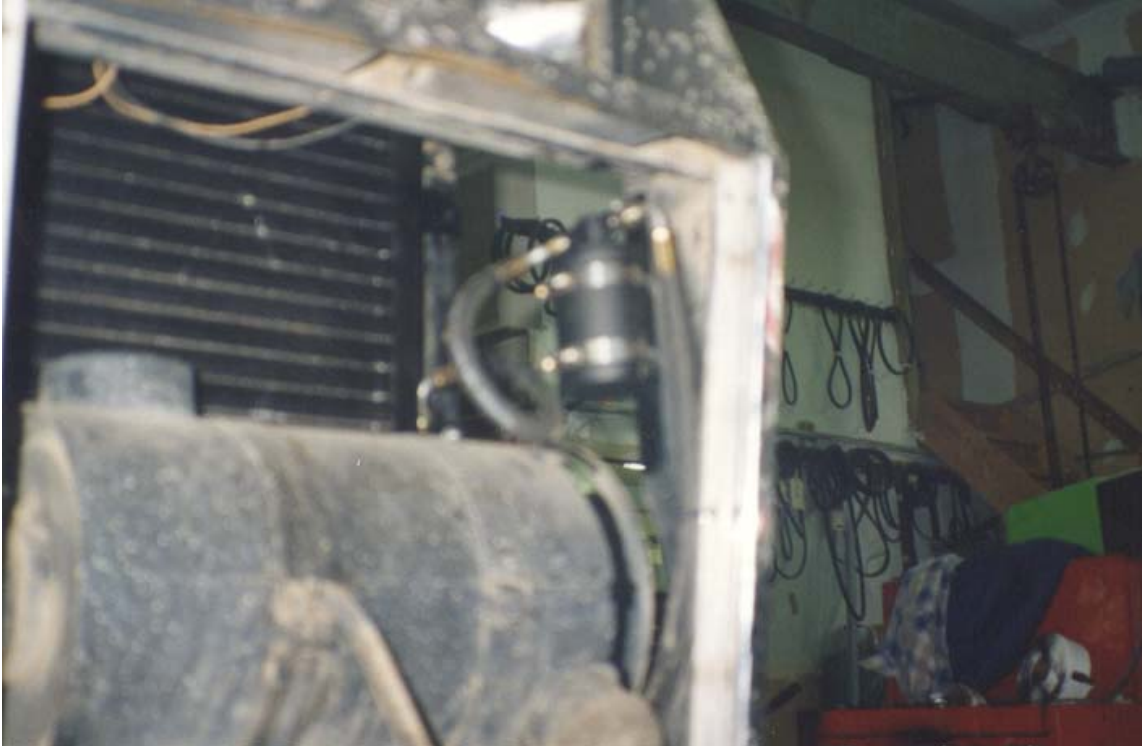
Drier in position in front of condenser.
